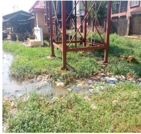
Plate 6: Poor sanitation at Ogida market
