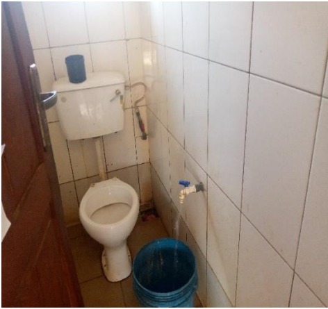
Plate 5: Flush toilet at Ogida toilet facility
